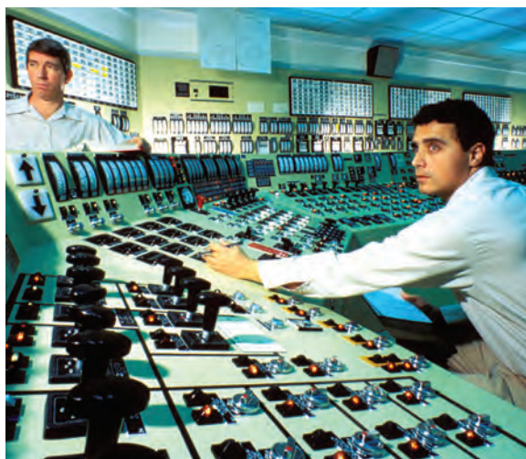
Nuclear power plant operators use computers and sensors in the control room to monitor the reactor.
